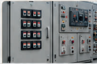
ELECTRICAL PANEL BOARD
